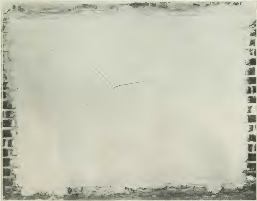
FIG. 19. CRACKS DEVELOPED IN SOLID PLASTER BOARD AND PLASTER PARTITION
